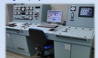
Engine Control Console
