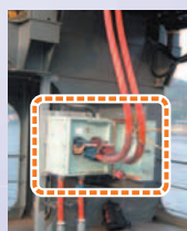
Ship side facility 船側設備
