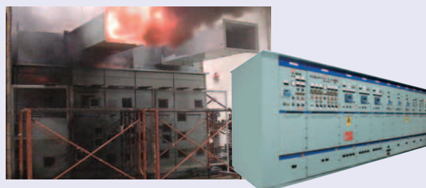
Arcing due to internal fault test HS21 内部アーク短絡試験
